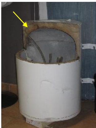
Picture 6. Water boiler (arrow pointing at insulation foam).
